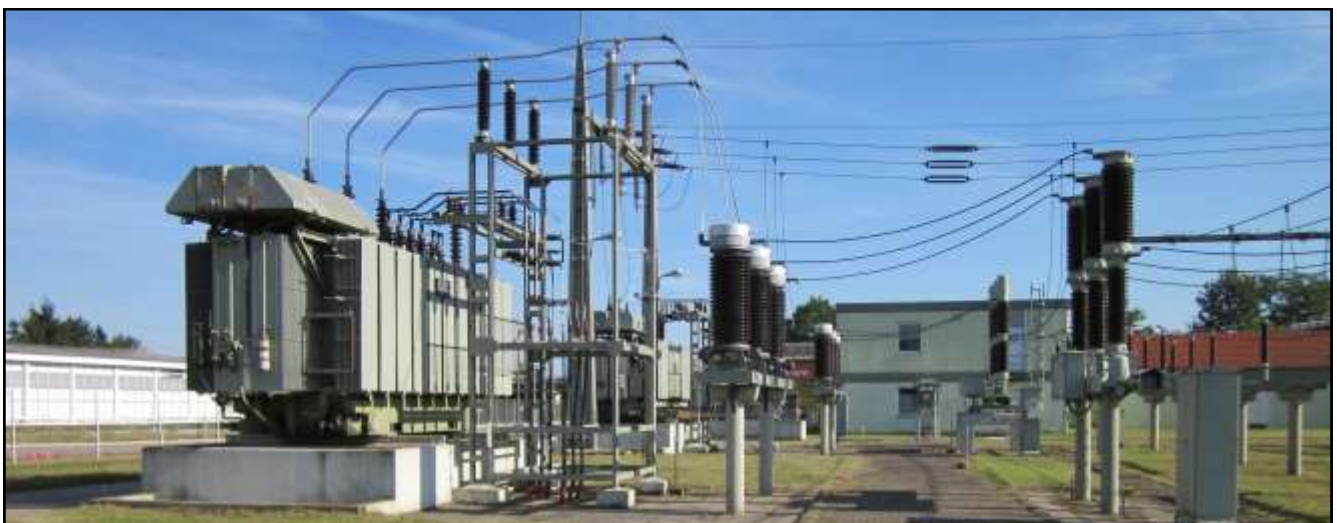
High Voltage Transformers
