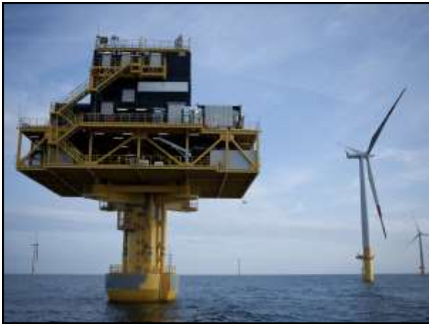
Converter substation offshore
