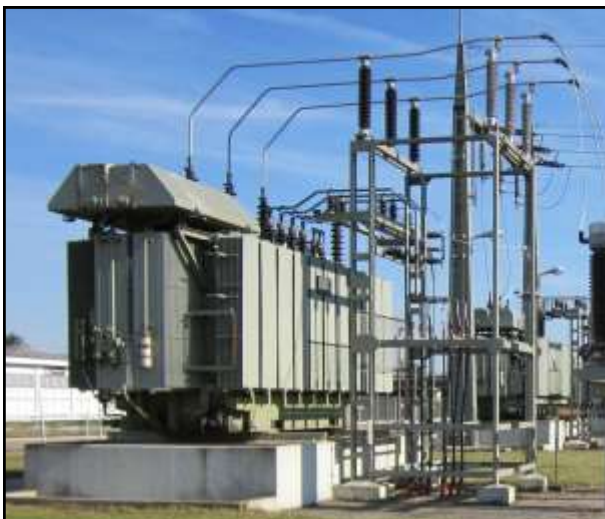
High Voltage Transformers / Smart Grids
